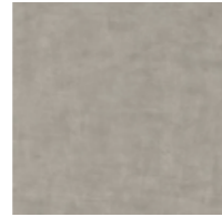
A00311 DISTRESSED CONCRETE
